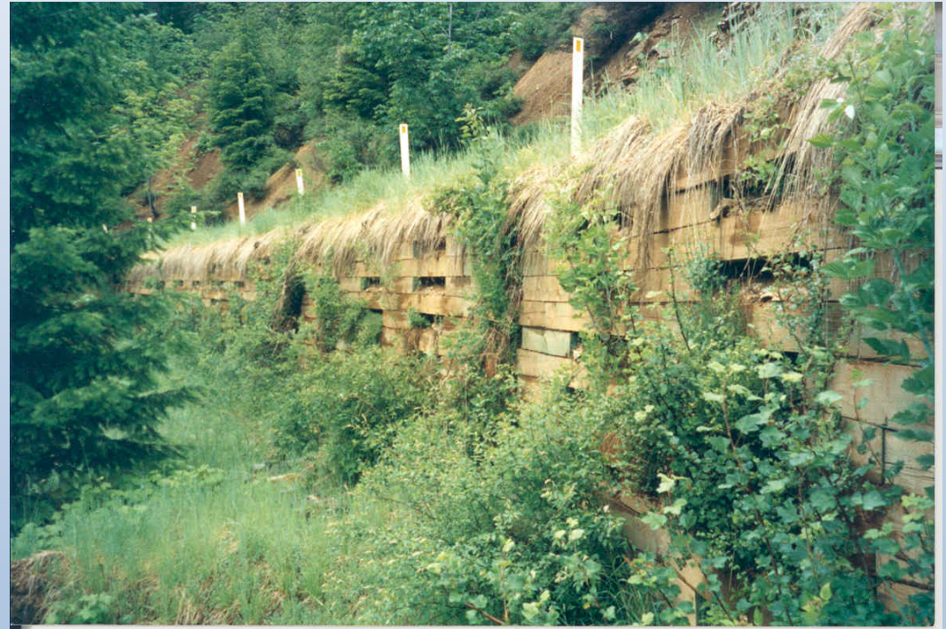
MSE Wall 3 Years after Construction. Happy Camp R.D. averages between 60 and 80 inches of precipitation per year
