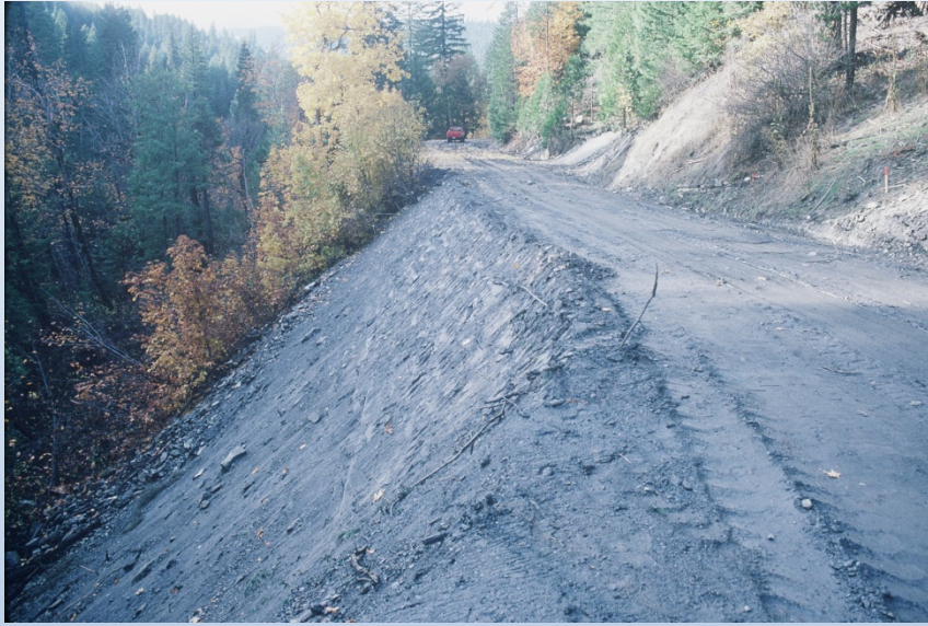
Reinforced Fill Just Completed and Before Erosion Control Mat Placed on Slope.
