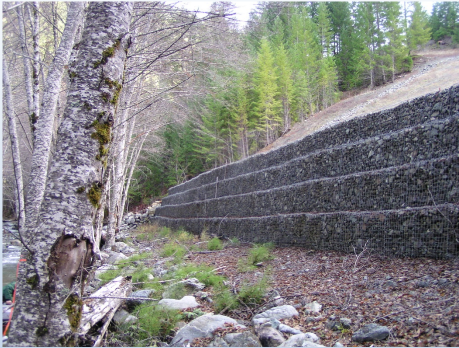
Gabion wall at reclaimed mine site on Klamath N.F. Region 5
