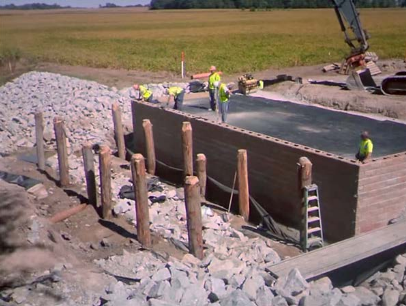
Photo Courtesy of FHWA
