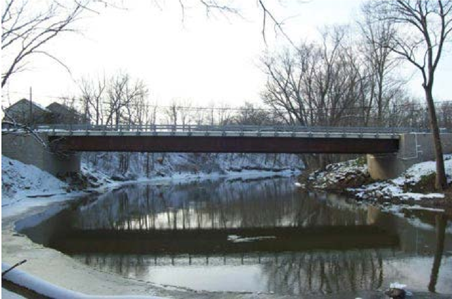
Photo Courtesy of FHWA
